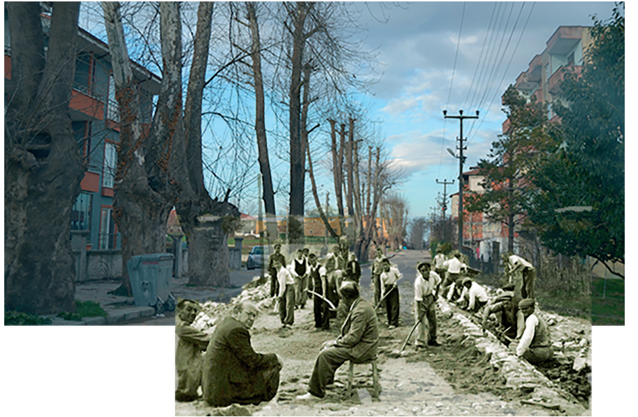
Figure 17. The road built by the village institute students between Area 1 and Area 2 – a comparative study by a photo collage of photographs from the construction period and 2020
