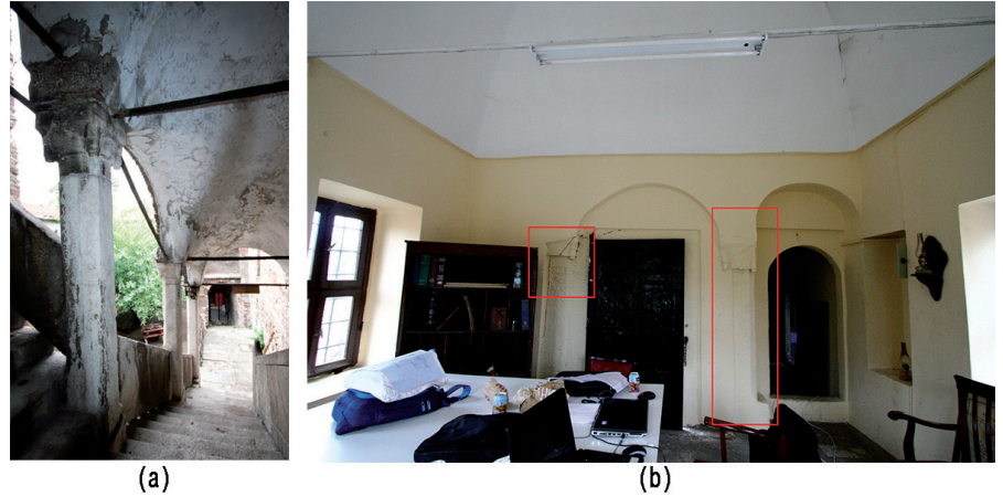
Figure 24. (a) The Columns at the Staircase, 2012. (b) The Columns Embedded in the Northeast Wall of the Room 201, 2012.
