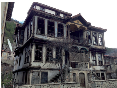
Figures 3, Figure 4 and Figure 5. Examples of registered historic houses in need of restoration. (General Directorate of Cultural Heritage and Museums, 2006)
