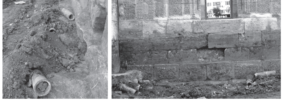
Figure 3. Terracotta pipes unearthed at the passage between Sivas, Izzeddin Keykavus I Hospital /Şifahiye and Çifte Minareli Medrese, found in situ at the foundation wall level of the medrese during 2011 restorations (Photos by the authors, 2011).
