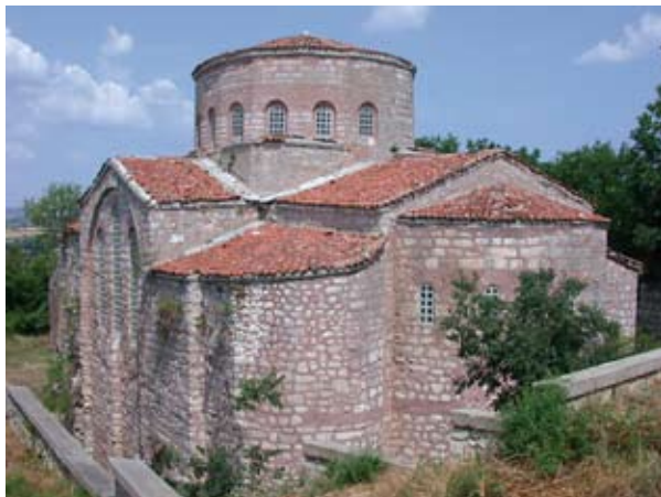
Figure 10. In the Small Hagia Sophia Church in Kırklareli stone damage was observed, which may superpose the heterogeneous distribution of different limestone varieties in the walls (at left, before turned into a mosque).
