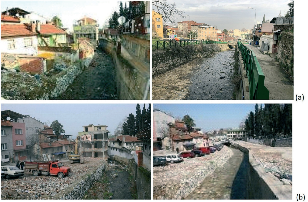
Figure 14. Before (a) and after (b) the rehabilitation process along the Cilimboz Valley due to the flood in 2010 (Bursa Metropolitan Municipality, 2024).
